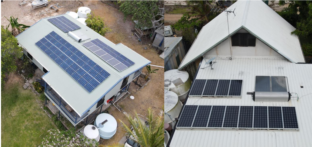
Figure 19: Professionally installed solar PV and solar hot water systems installed at Muralug
