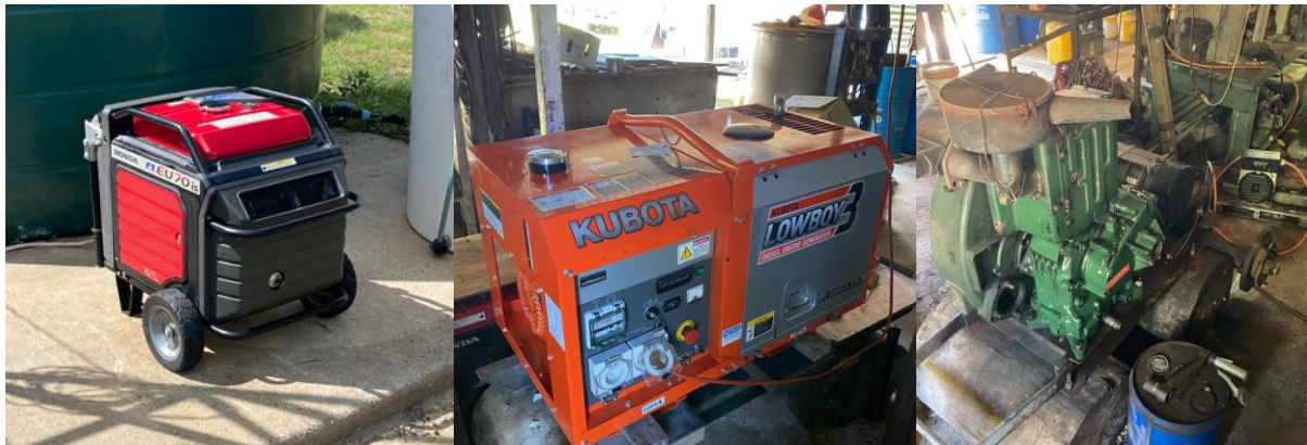
Figure 18: Typical small, medium, and large generators installed at Muralug.
