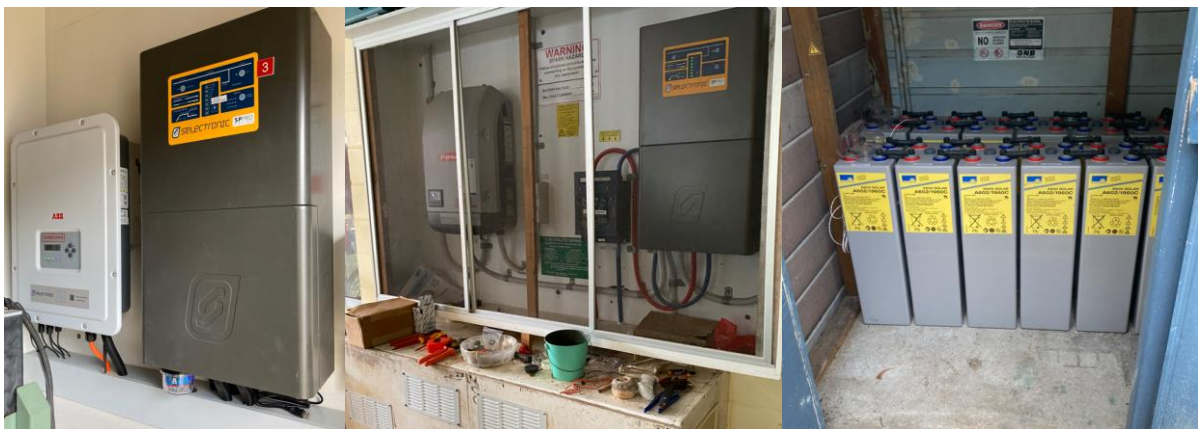
Figure 20: Professionally installed inverters and batteries installed at houses on Muralug
