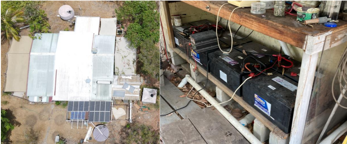
Figure 17: Non-professionally installed solar PV and batteries at Muralug
