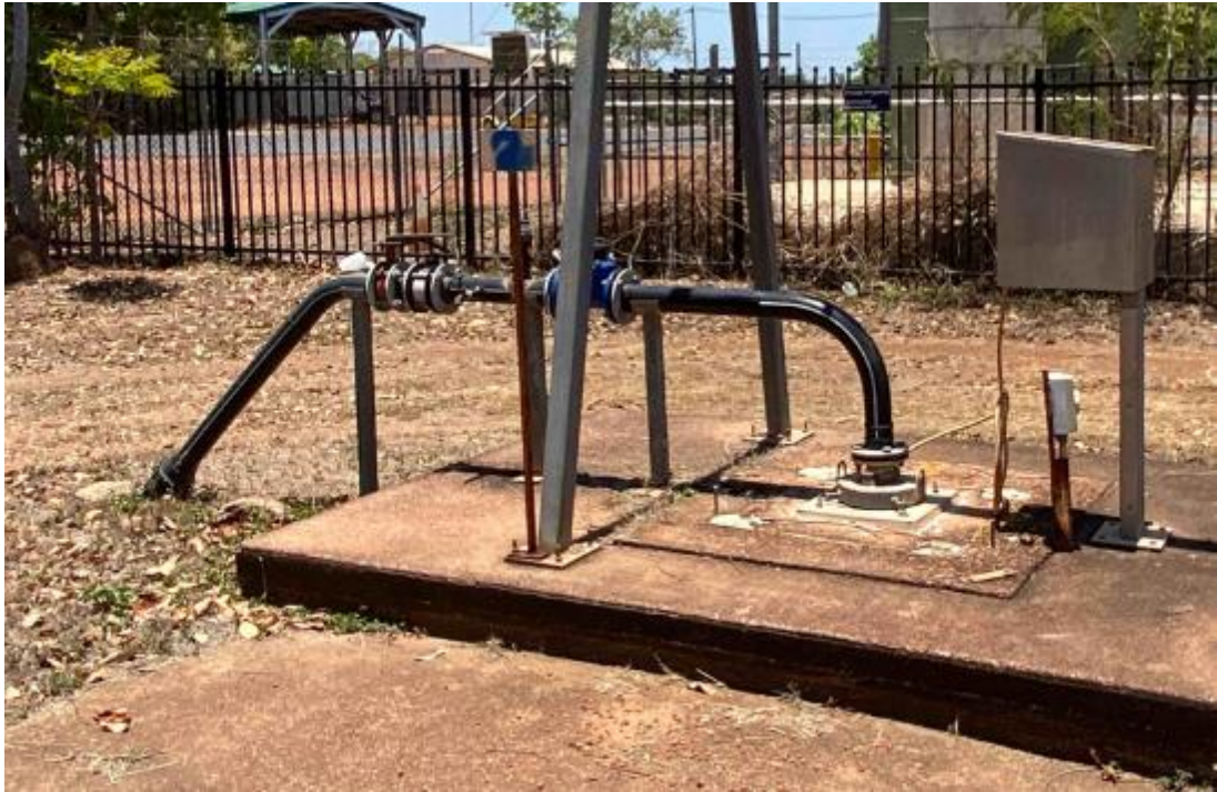
Figure 20: NASC water supply bore pump
