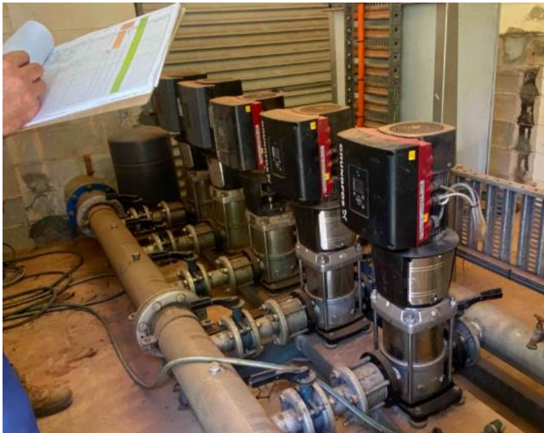
Figure 21: NASC water supply pressure pumps
