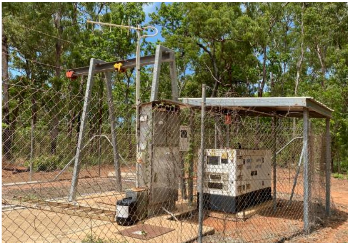
Figure 23: NASC sewerage pump station number 3 with standby generator
