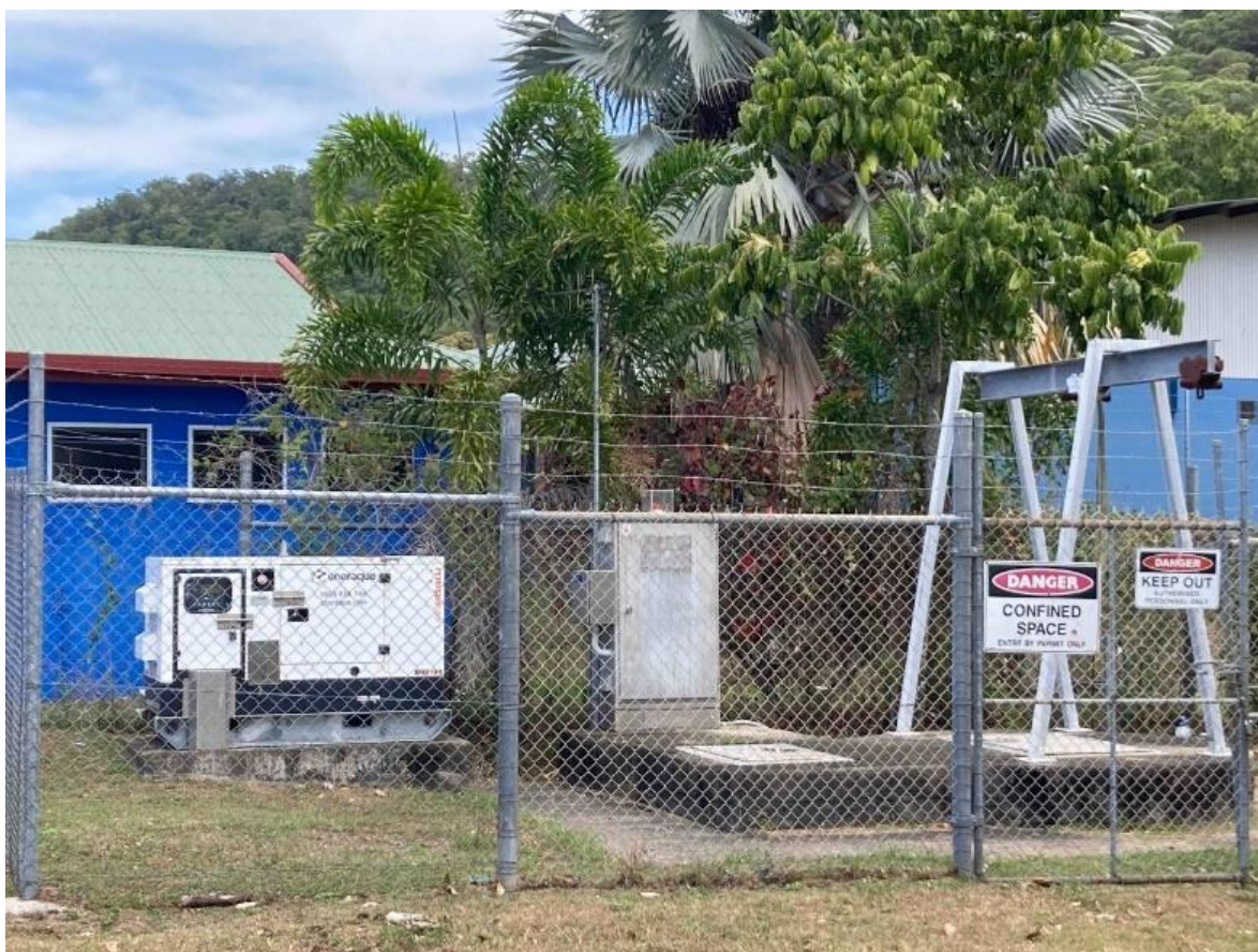
Figure 36 Typical sewerage pump station - Yarrabah
