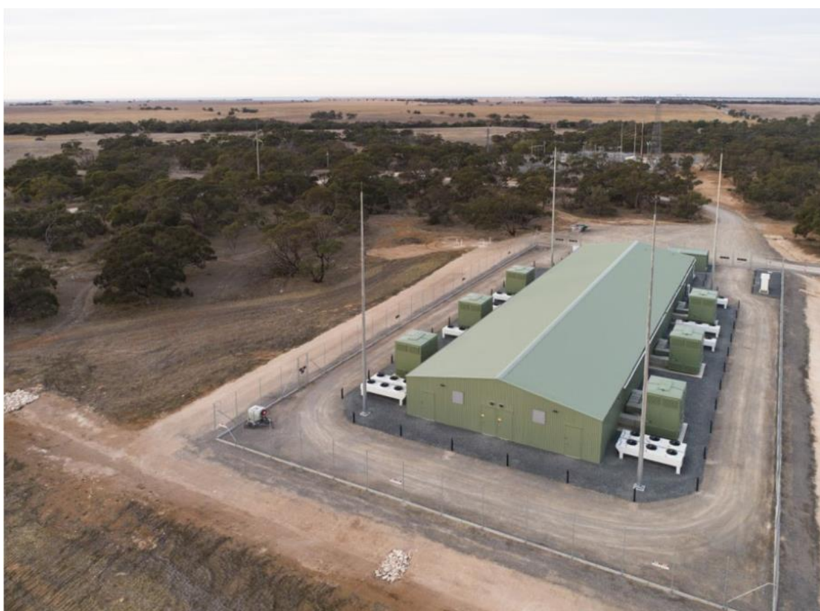
Figure 54 Dalrymple BESS facility 131
